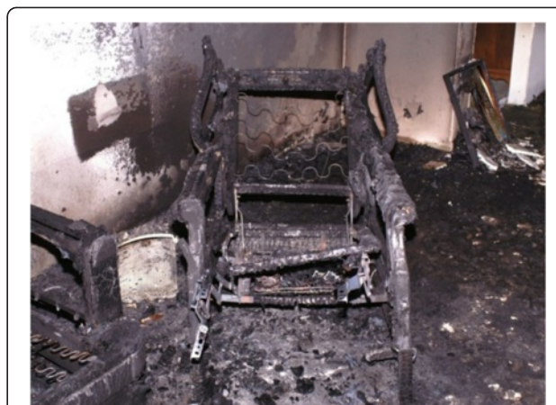
Fig. 14 Pre-fire Drywall Repairs Influencing the Post-fire Visible Damage to the Wall (fire origin located along front of chair-fire test conducted at EKU by author)
