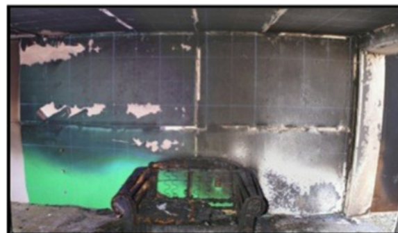
Fig. 13 Ventilation-Generated Fire Pattern near open doorway (fire origin located across room-fire test conducted at EKU by author)
