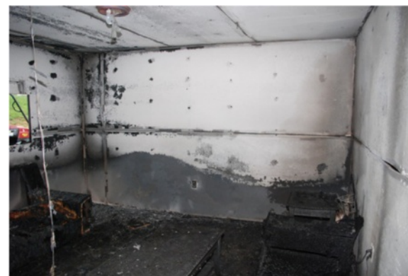
Fig. 12 Upper Layer-Generated Fire Pattern (fire origin was located along adjacent wall-fire test conducted at EKU by author)
